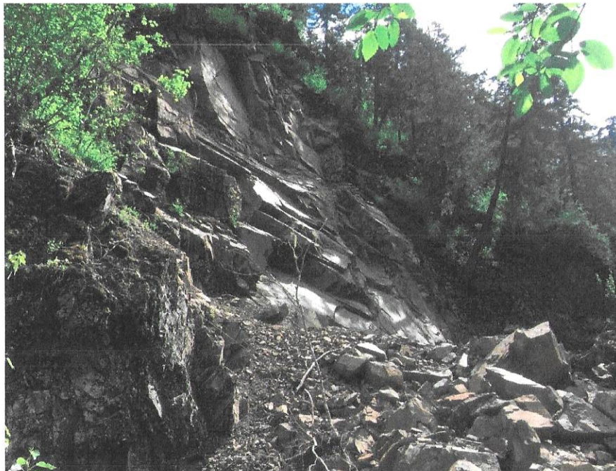
Photo 2. Exposed rock face, standing at 70-75°. The dip of the rock strata is coincident with the slope, rendering it unstable, particularly for individual rock fragments. The hazard warrants construction of a protective berm.
